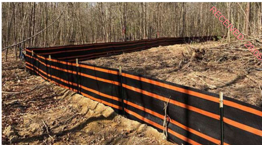
Figure 7. Example of Silt fencing.
